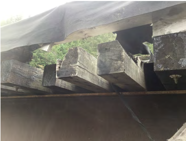
2 untreated ties at right bank untreated and in poor condition
