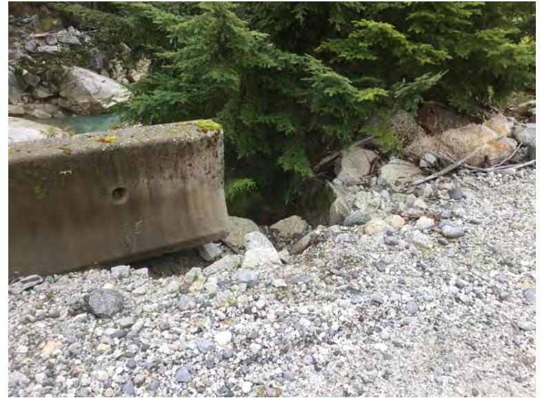
Eroding fill on downstream right approach
