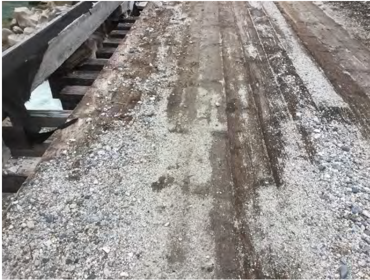
Rotting deck planks
