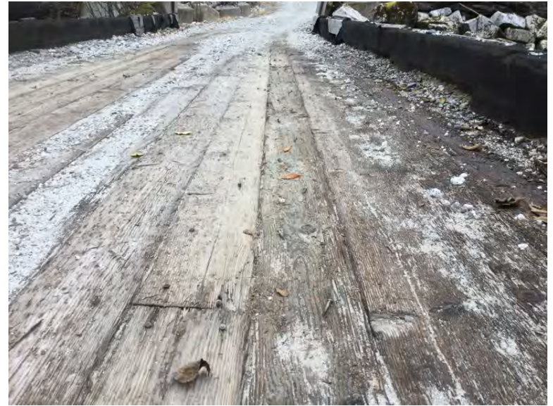
Rotting deck planks
